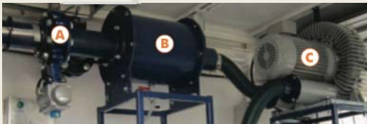
A) Atmospheric valve B) Accumulator C) Regenerative blower
